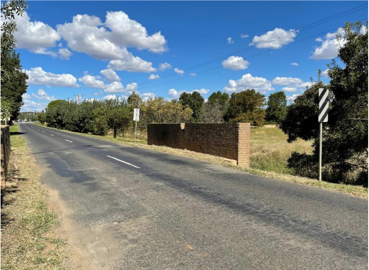
Figure 2-15: Lord Street Bridge showing current dilapidated state
